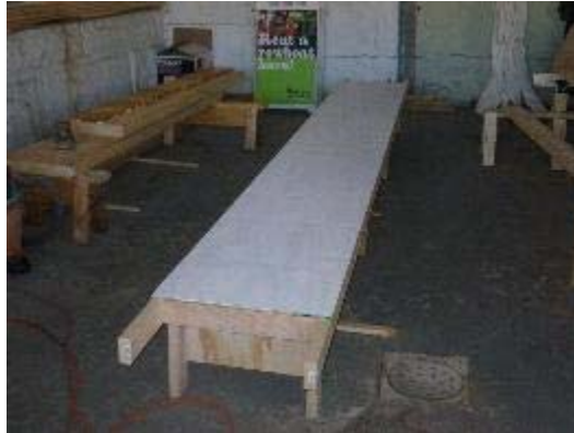
Building form for the new boats will be set up on this new strongback
